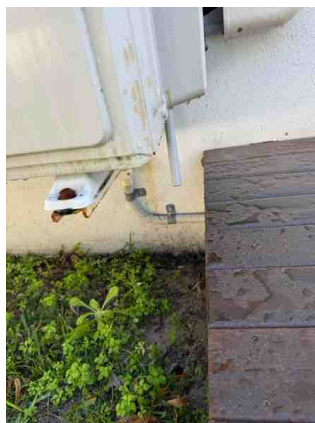
We recommend that air conditioner motor be drained to storm water.
